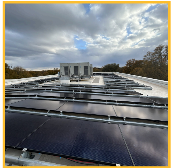
Rooftop Solar at Town Hall
