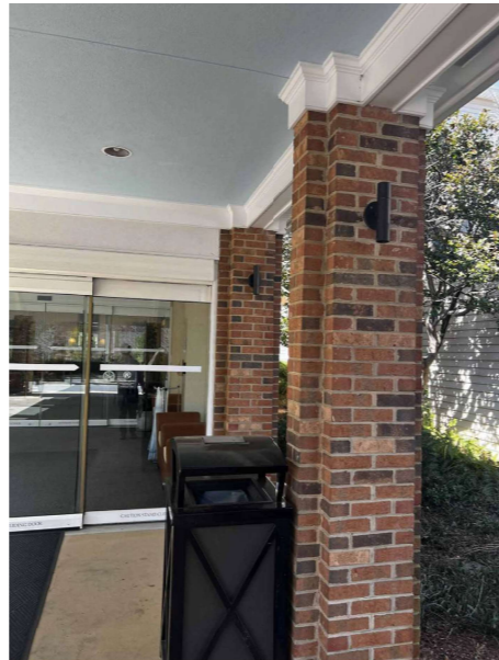
B. COMMONS ENTRY - ENTERING VESTIBULE WE ARE MATCHING THE LIGHT FIXTURE AT THE MAINTENANCE BUILDING
