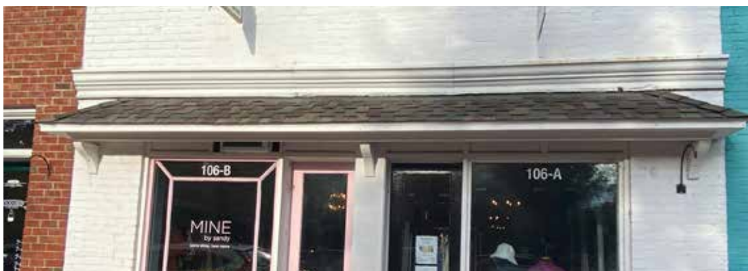
This is an example of an added mansard roof over a storefront. A more appropriate treatment may have been a fabric awning.
