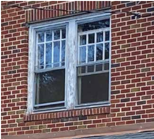
Lack of proper maintenance of wood features may result in moisture problems such as on these windows.
