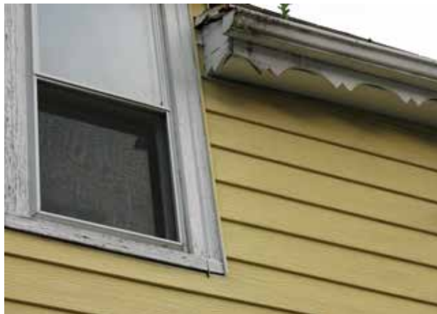
This example shows the visual impact of added vinyl siding on the character of the building. Maintenance and paint is needed on the historic wood trim.
